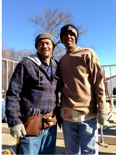
Tsegaye (pictured, at left, working at a Habitat build site towards his required sweat equity hours).
