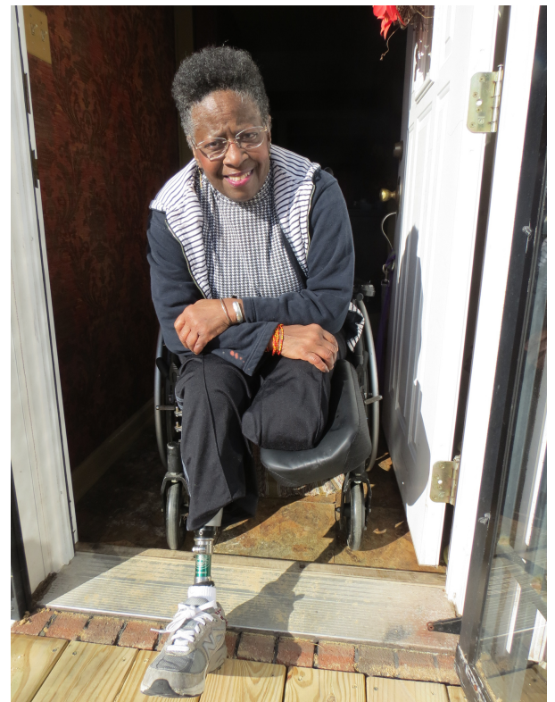
Rosaland watches as Habitat Susquehanna's Repair Program builds an accessibility ramp for her home.
